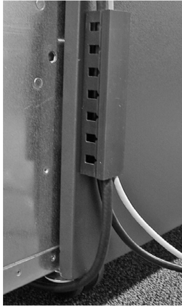
Figure 25. Back Panel Long Cable Ducts for A12 SMS
